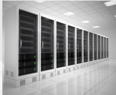
Fibre & Copper Structured Cabling System
